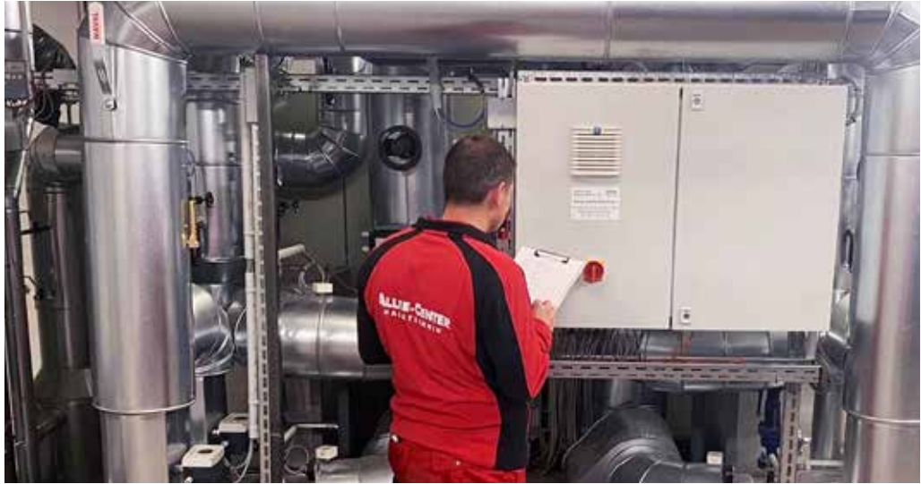
District heating station of the Allee-Center, Magdeburg
